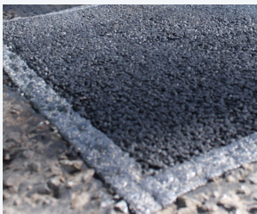
Make sure damaged flooring is repaired
